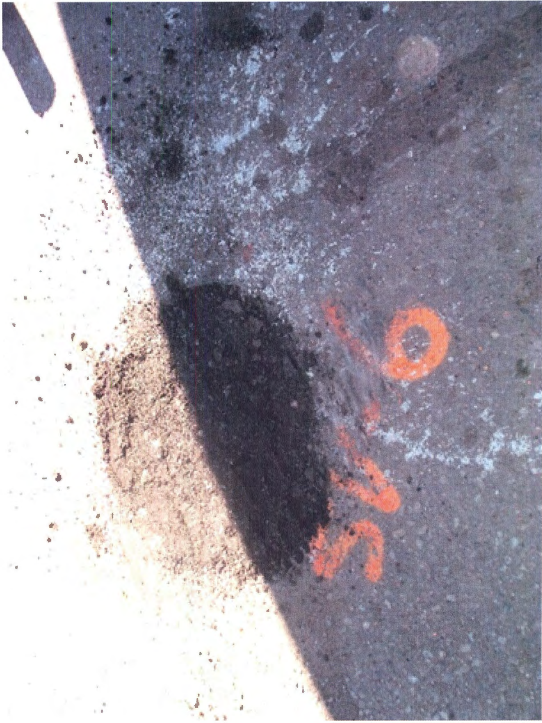
Photos: Plugged SVE-6 – well casing and vault left in place. Gramms 66 site in Quinter, Kansas MILCO Project No. M269-P1-01
