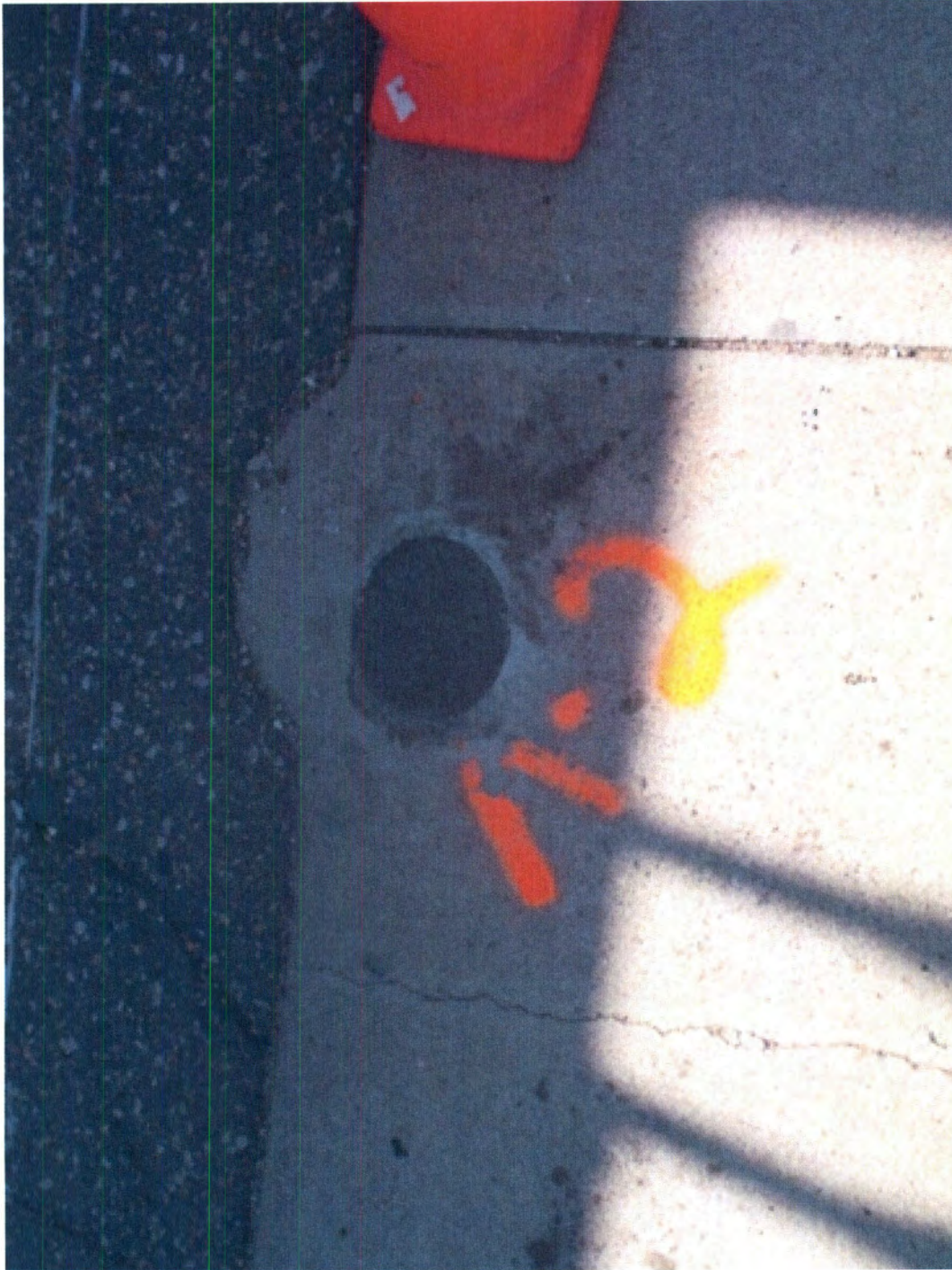
Photos: Plugged AS-2 – well vault left in place Holiday 66 site in Hays, Kansas MILCO Project No. M273-P8-01
