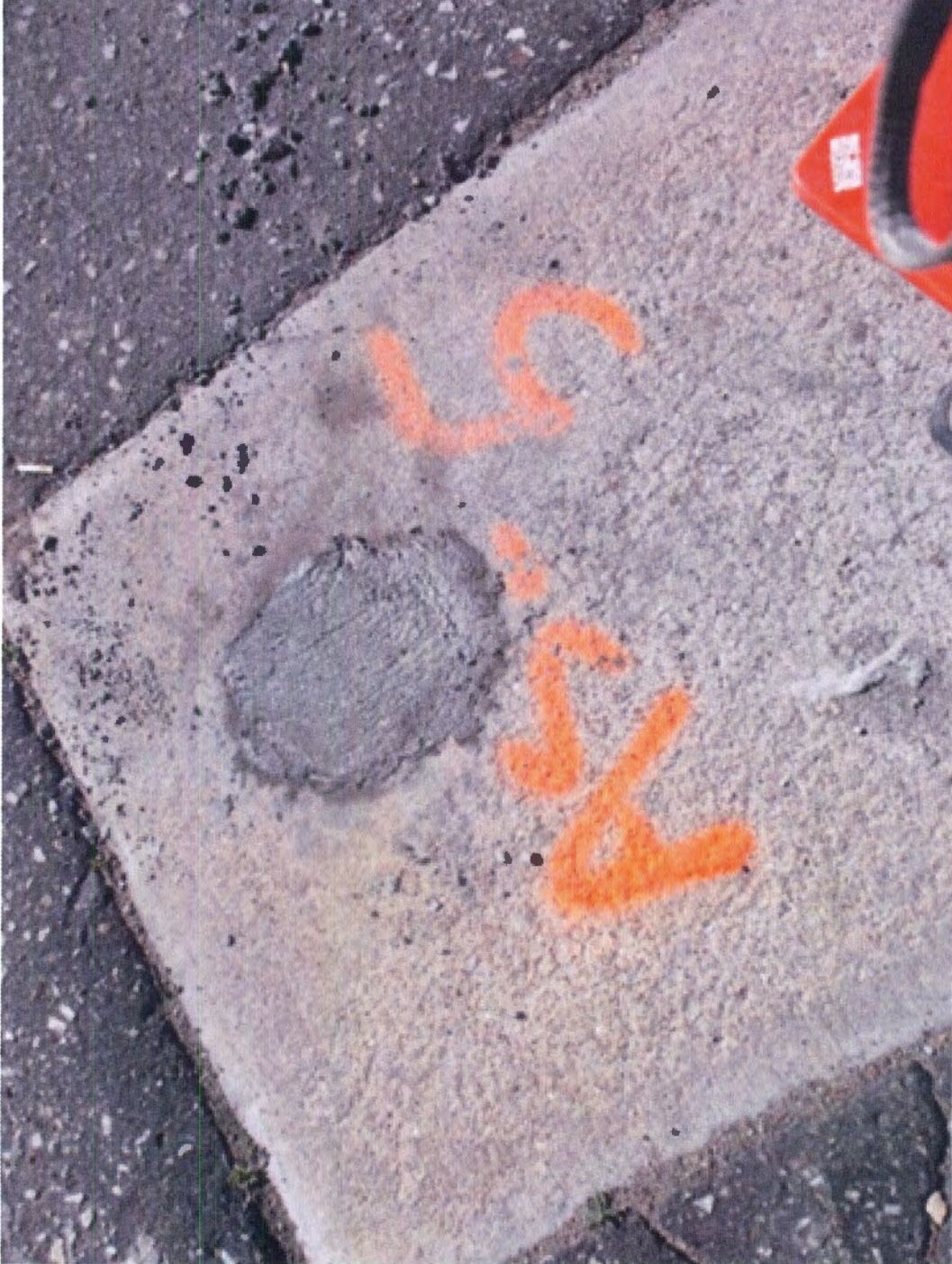
Photos: Plugged AS-5 – well vault left in place Holiday 66 site in Hays, Kansas MILCO Project No. M273-P8-01
