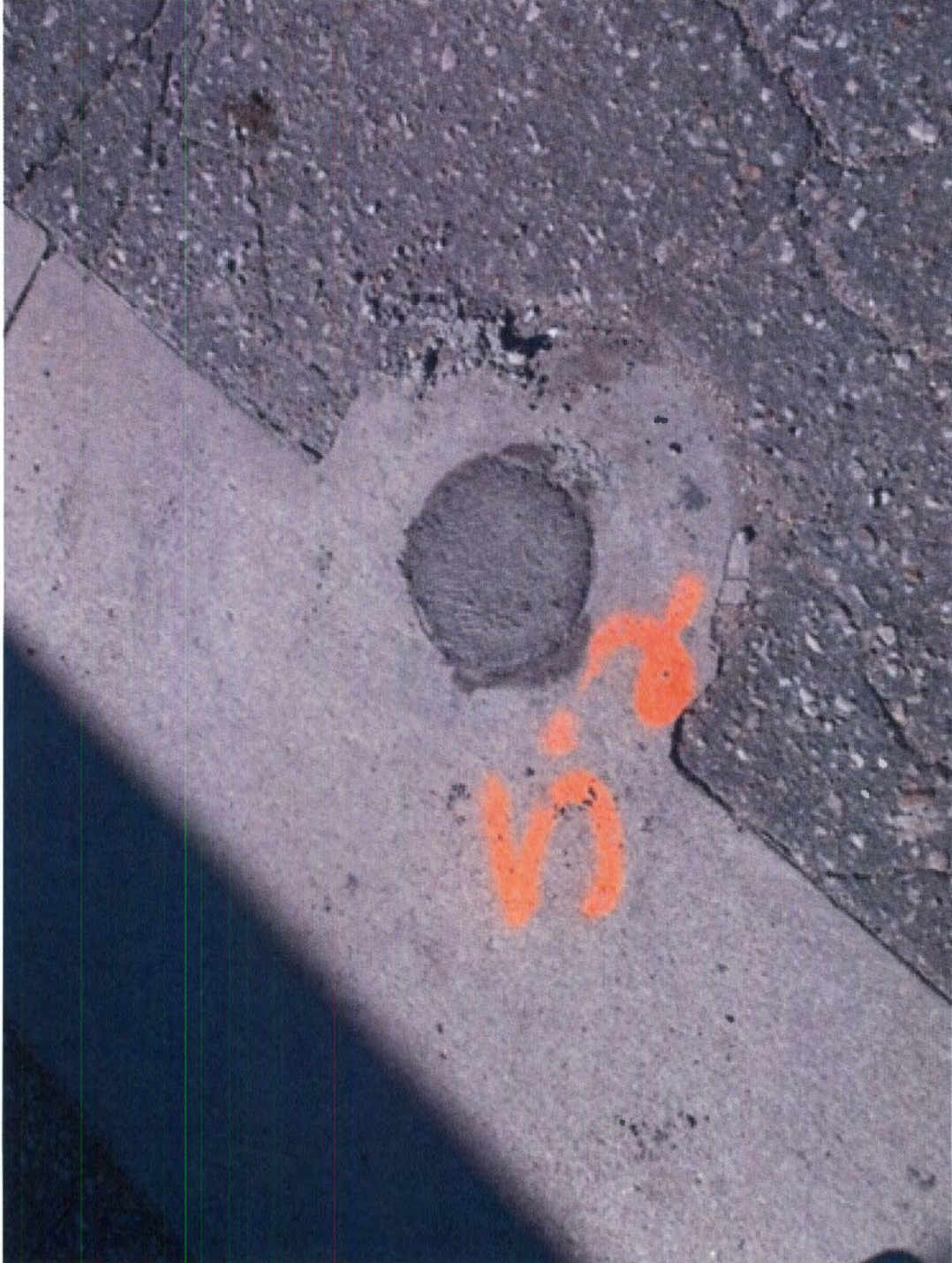
Photos: Plugged SVE-2 -- well vault left in place Holiday 66 site in Hays, Kansas MILCO Project No. M273-P8-01
